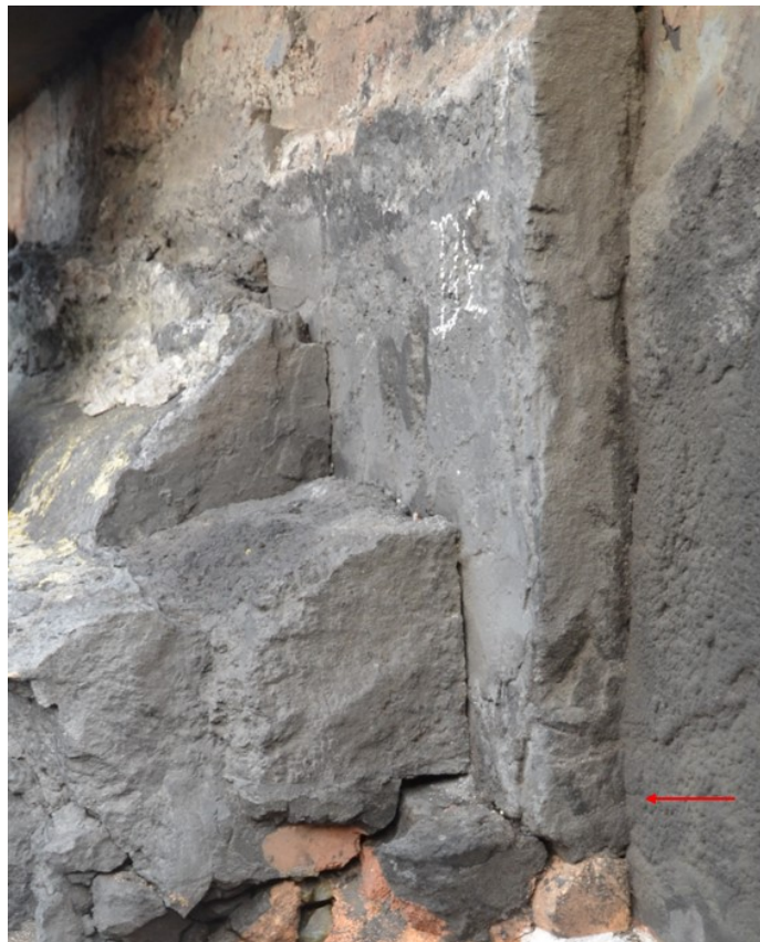
Figure 5. Reacted refractory brick at base of SiC on the shell side.
