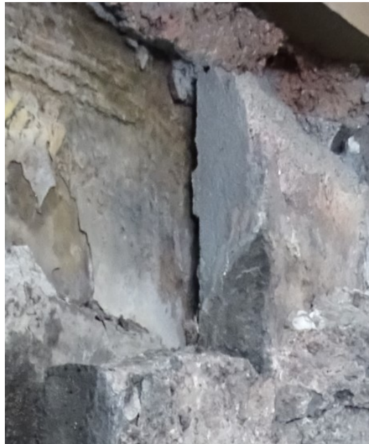
Figure 4. Air gap formed between SiC slab and steel shell.
